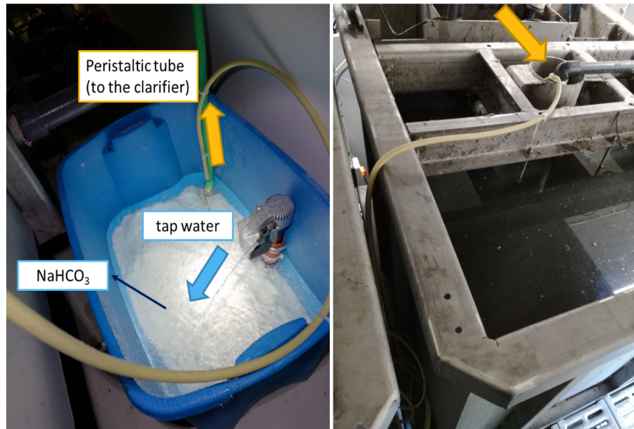
Figure 4.27: Alkalinity dosing set-up at the pilEAUte using a saturated sodium bicarbonate solution. Left: the dosing basin, right: dosing location on the primary clarifier
