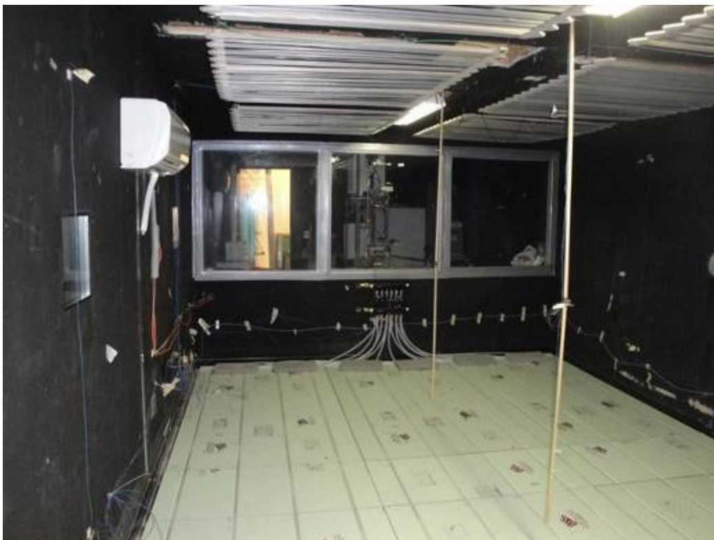
Figure 28 Experimental test chamber with radiant concrete floor loop, before installation of the concrete layers
