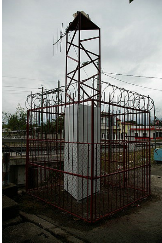
Figure 7.1: 5 Meter Antenna Tower with Security
