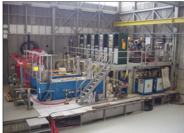
Figure 2: MTE kicker generators.
