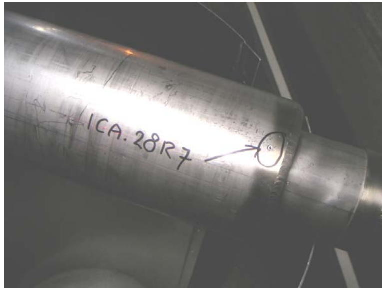
Figure 10 – Accidentally drilled and pop-riveted F line compensator.
