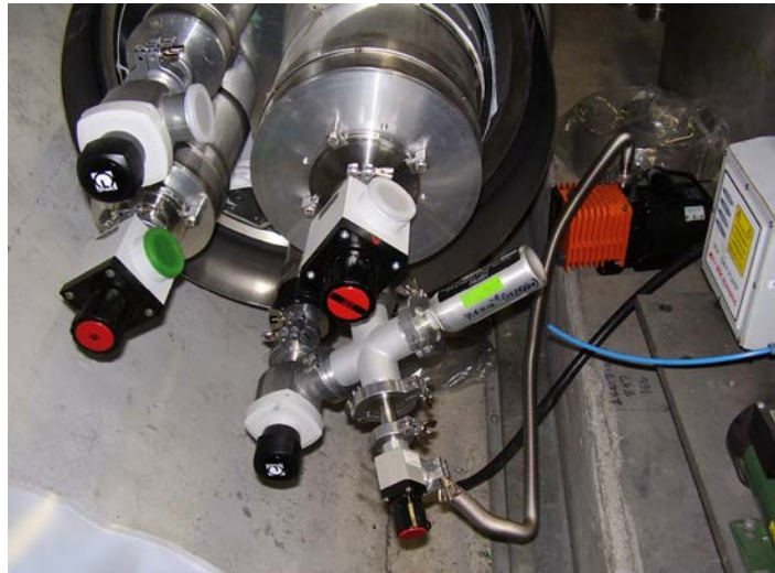
Figure 6 – Pump-out tools acting as plugs installed on the process lines. The tool on line F (bottom) is equipped with a reference leak for a system calibration
