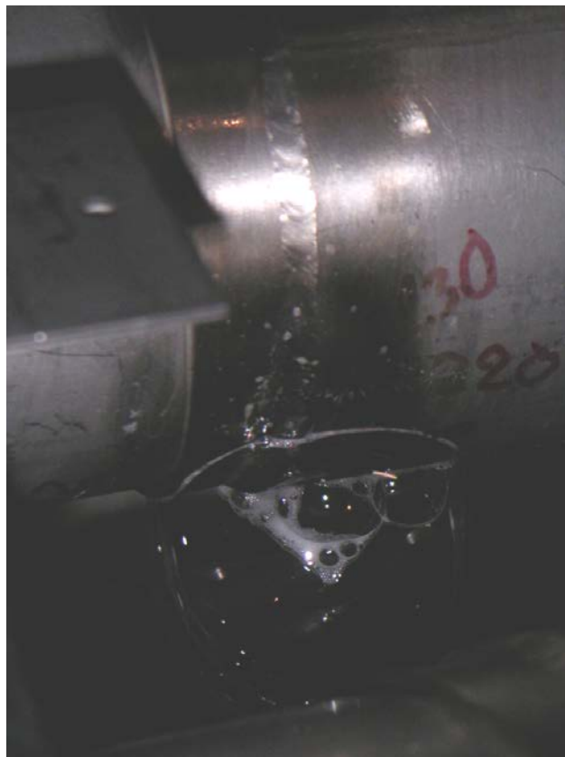
Figure 5 – Localisation with bubble spray of a large leak in the interconnection weld of a process line.
