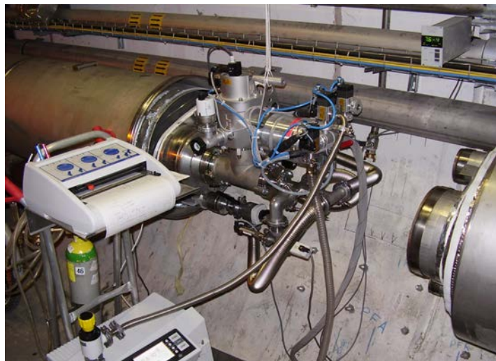
Figure 7 – Pump-out tools installed on the process lines. The tool on line B (largest diameter) is equipped with a manifold connecting the turbomolecular pump to all process lines in parallel.
