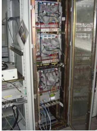
Fig. 51: The Elettra horizontal, vertical, and longitudinal feedback processors
