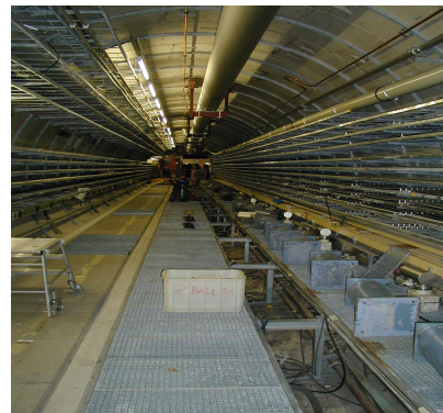
Figure 5: HERA tunnel after removal of the old hardware in the interaction region N/S.
