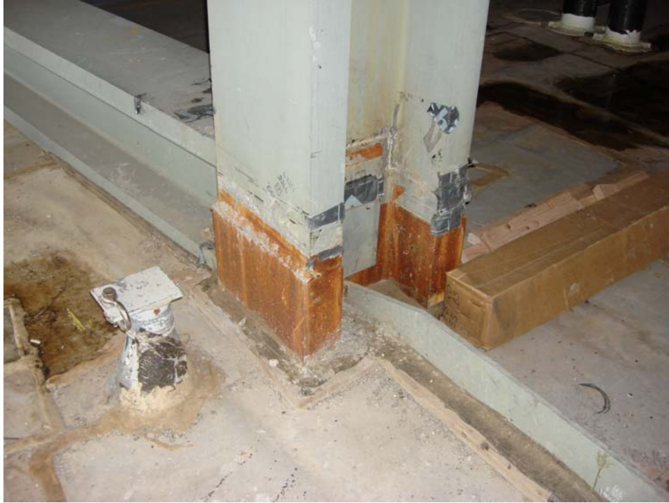
Figure 3.10: Welded connection of the new and existing structure at the Phase 1 roof level (Source: Author).
