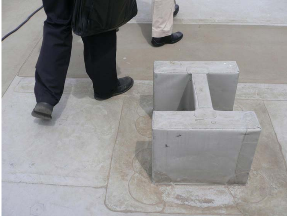
Figure 3.9: Top of Phase 1 column extended through the roof slab and waterproofed to facilitate a connection for the Phase 2 expansion (Source: Goettsch Partners, 2008).
