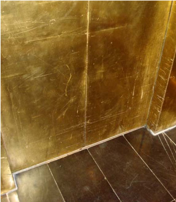
Photo 6: Photo taken by Damien B. Chaviano on June 23, 2008. There is no air conditioning in either the hallways or elevator. From June 19 through June 22, three of the four elevators were out of service.
