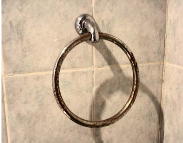
Photo 4: Rusty towel ring in hotel room. Photo taken by Damien B. Chaviano on June 23, 2008. The Havana Libre is described as a five star hotel. This photo of a rusty towel ring questions the five star rating, and suggests that very few renovations have been made.
