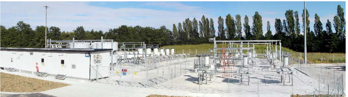
Figure 6: Photo of the SVC installation
