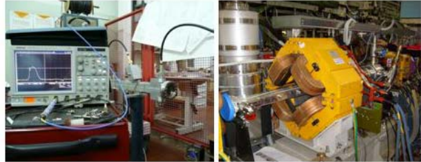
Figure 7: New fast injection kicker under test (left) and installed on the electron ring (right).
