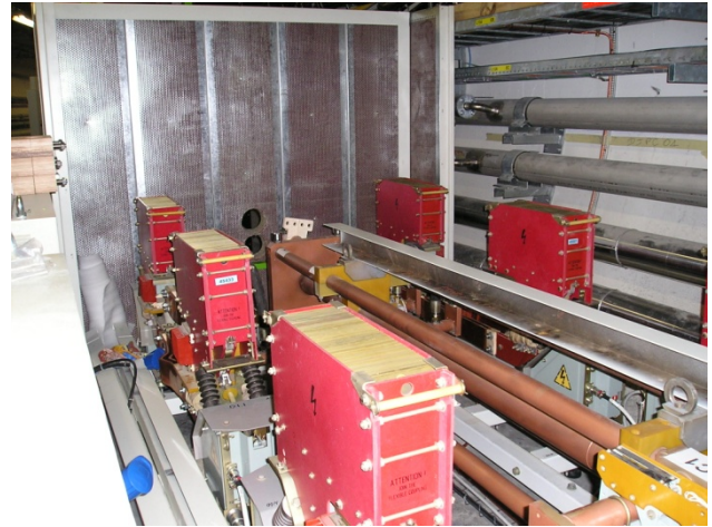
Figure 1: A view on the 13 kA switch unit for the dipoles.
