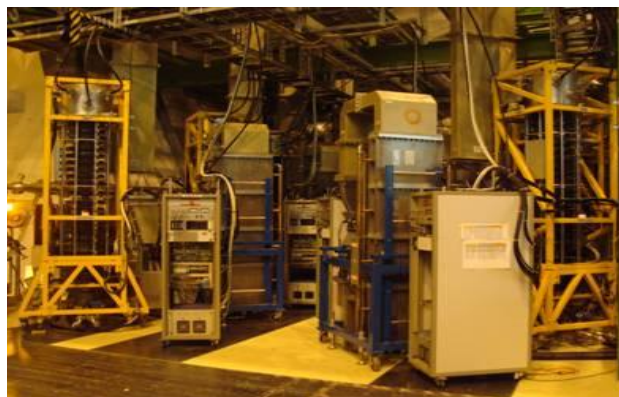
Figure 2: Klystrons, Power Equipment and Control Racks in the UX45 Cavern.
