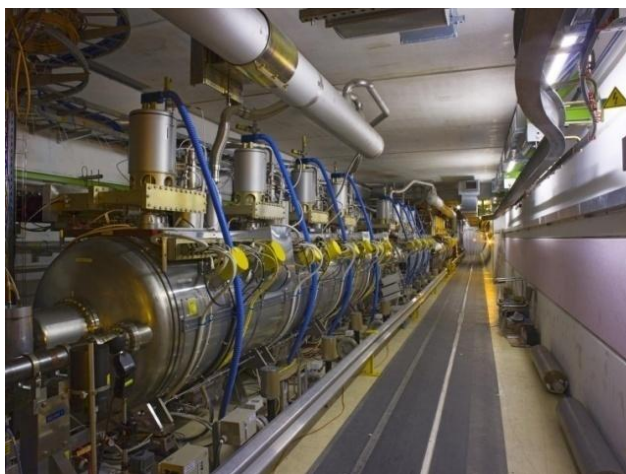
Figure 1: RF Cryo-modules in the LHC tunnel at IP4.
