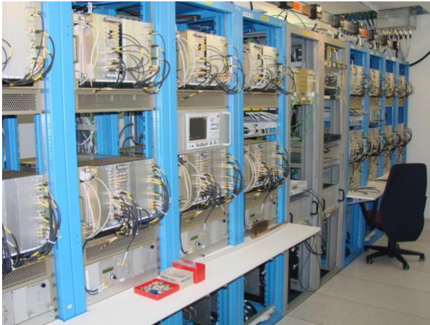
Figure 4: Cavity Controllers in UX45 Faraday Cages.
