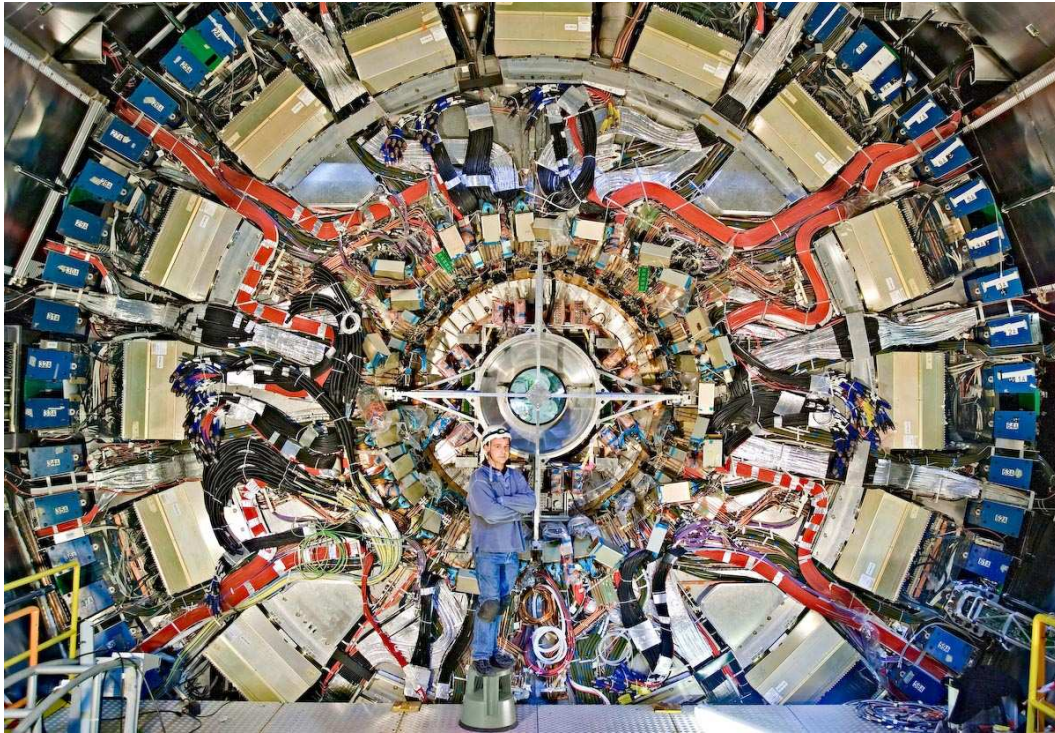
Figure 5.6: This picture of the services in the transition region (SIDE A) highlights the complexity and diversity of the materials to be described. Note the intricacy of the routing of services.
