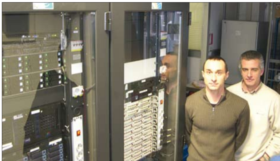
Massimo Nuccetelli (left) and Fabio Pellegrino, two of the technicians who helped in the realization of the new Rome centre, standing by the two currently installed CMS racks.
