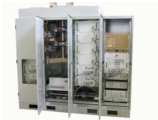
Fig. 5: [6 kA, 8 V] power converter
