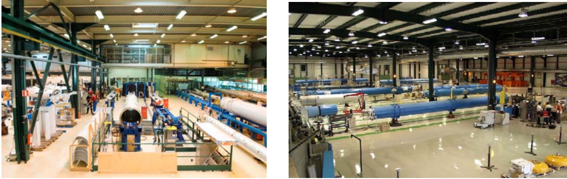
FIGURE 1. Pictures of the assembly halls of the LHC Short Straight Sections (left), dipole cryostats (right) at CERN.
