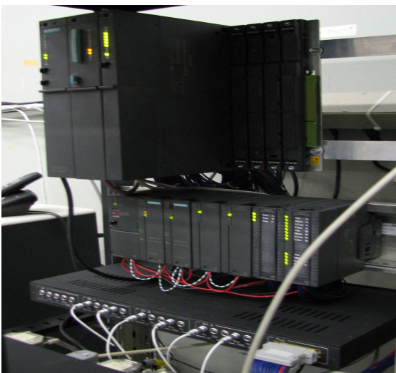
Figure 6: Photograph of the ESS installed and running in the ECAL Integration Area
