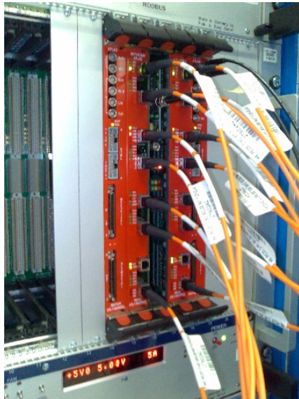
Figure 5 : The ROD Bus, showing the five boards mounted on the VME Crate in USA-15 room, one ROD, two Sector-Logic/RX and two MUCTPI-Interface boards.
