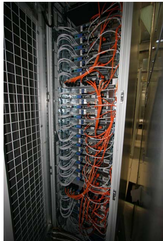
Figure 7: One RUBU rack fully cabled
