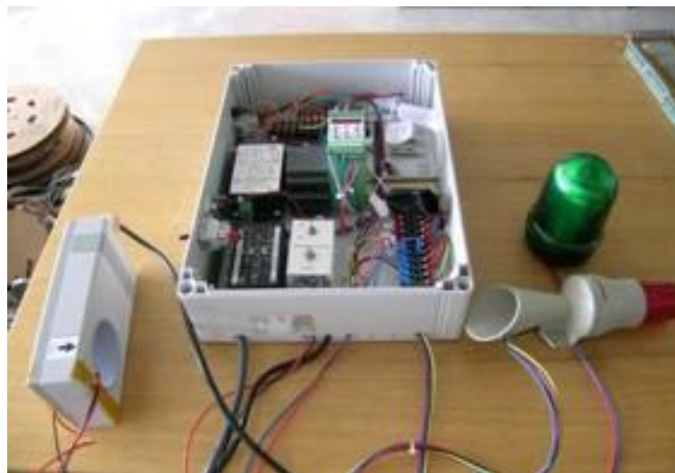
Figure 30: grounding monitor with ICPT, alarm and control system.
