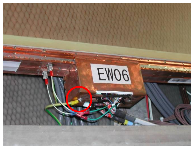
Figure 44: Faraday cage ground connection.
