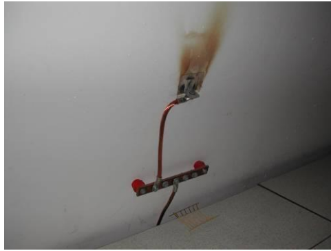
Figure 4: Grounding bar in USA15.
