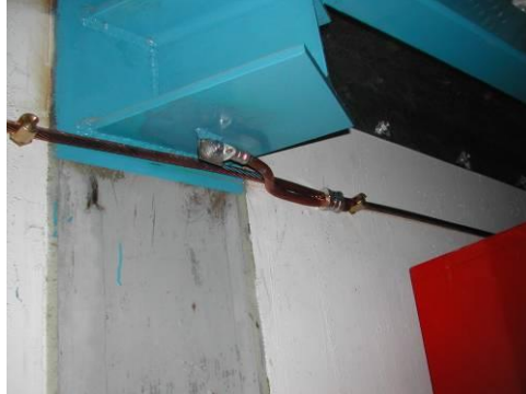
Figure 12: Grounding of the HO and HS structures.
