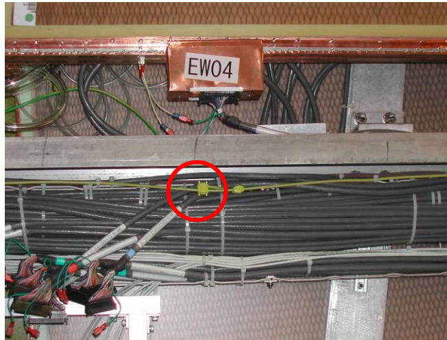
Figure 45: Tap connection of the ground wire.
