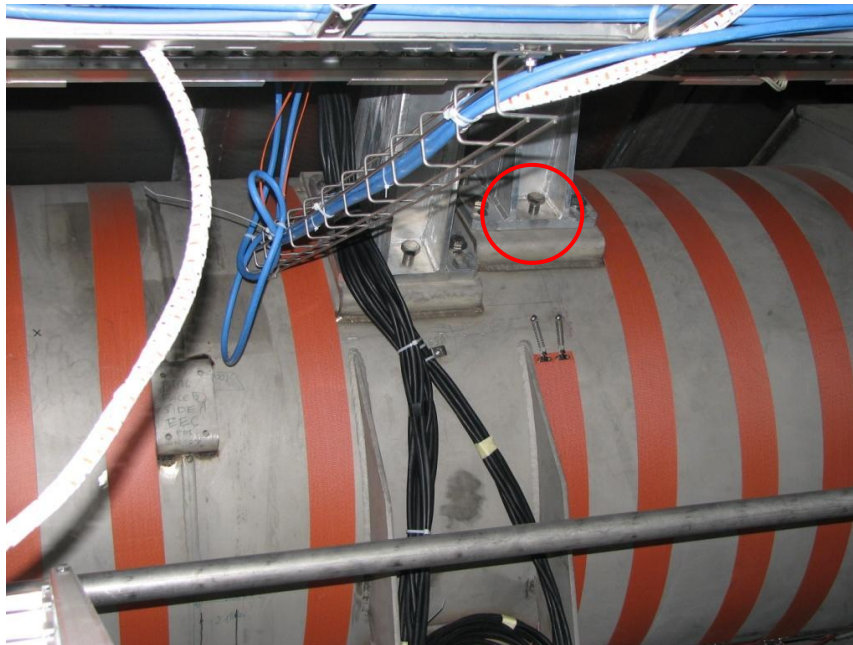
Figure 51: M15 link point of the grounding cables on the BT vacuum vessels.
