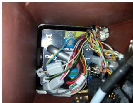
Figure 7: The inside of a finger with the services exposed.
