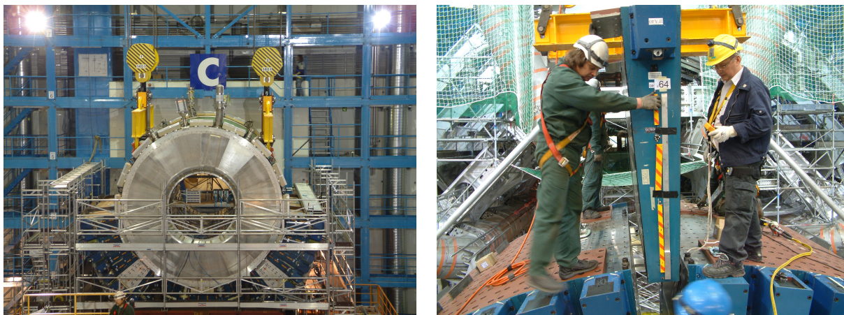
Figure 24: Installation of the barrel cryostat in the ATLAS cavern (left). The installation of the final TileCal module in the EBC cylinder (right).
