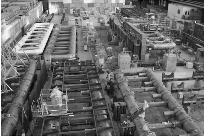
Fig. 2. View on the assembly and test area at a certain moment of assembly in February 2005. A few coils are already installed into the vacuum vessels. One cold mass is prepared for integration. One coil is in the X+ test bench. Being part of the production schedule a delay in the might affect the overall planning.
