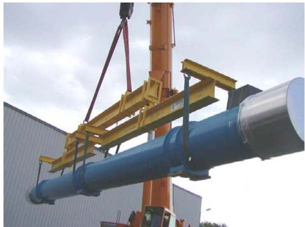
Figure 1: LHC cryodipole during handling with mobile crane. A double rotating spreader is used to guarantee the correct repartition of the loads as required
