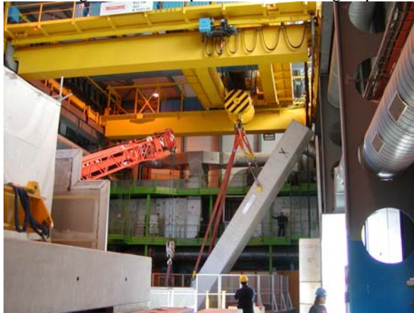
Figure 3: Tilting manoeuvre into PX85 shaft by means of coordinating building overhead crane and mobile crane
