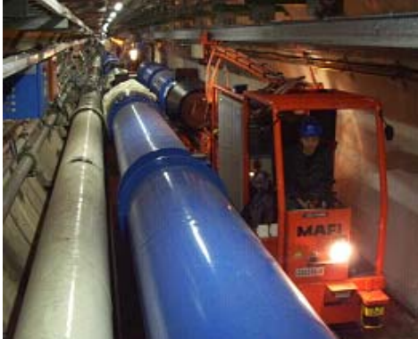
Figure 3: LHC tunnel with, from left to right: the cryogenic line, an installed and a transported magnet.
