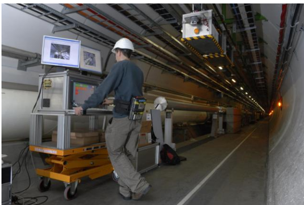
Figure 2: Functional testing of TIM in the LHC tunnel
