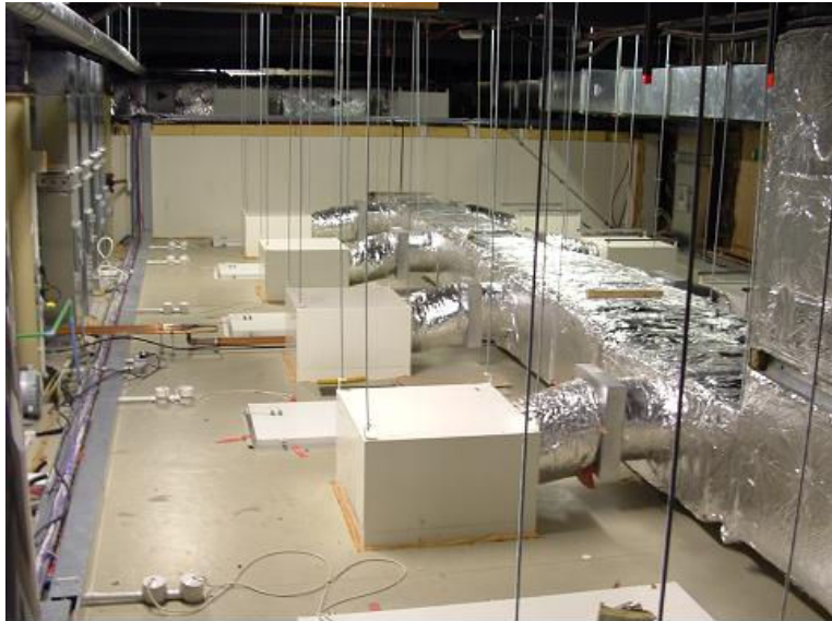
Figure 8: View of some of the plant room above the LHCB. Leaks in this area can damage equipment below.
