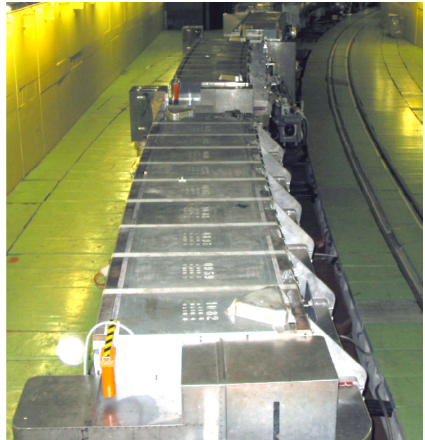
Figure 4: PS main magnet units. The ACEM BLM detectors are the orange cylinders mounted on top of the magnets.
