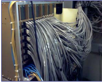
Figure 2 308 LVDS cables installed at the back of the backplane
