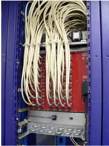
Figure 7: Cables into the RCT in the MTCC counting house.
