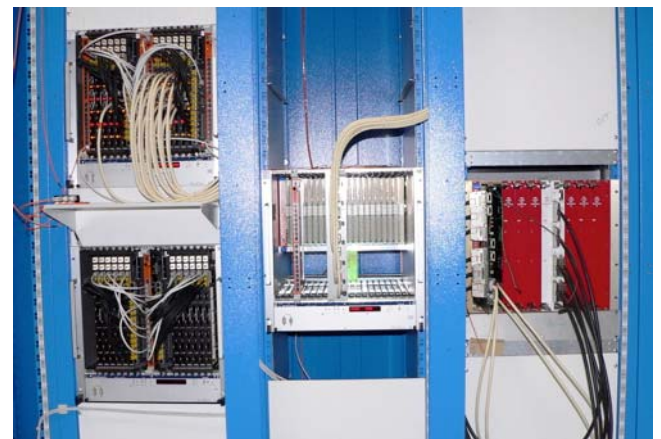
Figure 4: Front of the HCAL (right), ECAL (center), and RCT (left) racks at the integration facility. The top crate of the HCAL has the 19 cables attached to SLBs mounted on HTR cards. The ECAL rack has the TCC with SLBs and cables. The RCT has 6 cables (black) from the JSC to the JCC, and two cables (beige) from the CCC to the JCC.
