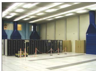
Ducts and grills provide cold air directly to computer air intakes.
