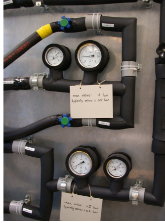
Figure 29: Pressure gauges at the cooling system of the early setup.
