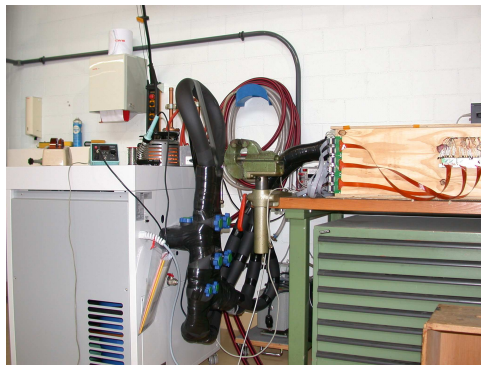
Figure 18: Chiller (left) connected to the test box with insulated tubes.
