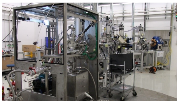
Fig. 8. Picture of the LiLiT-2 system installed at SARAF new target room with the frame of the containment vessel
