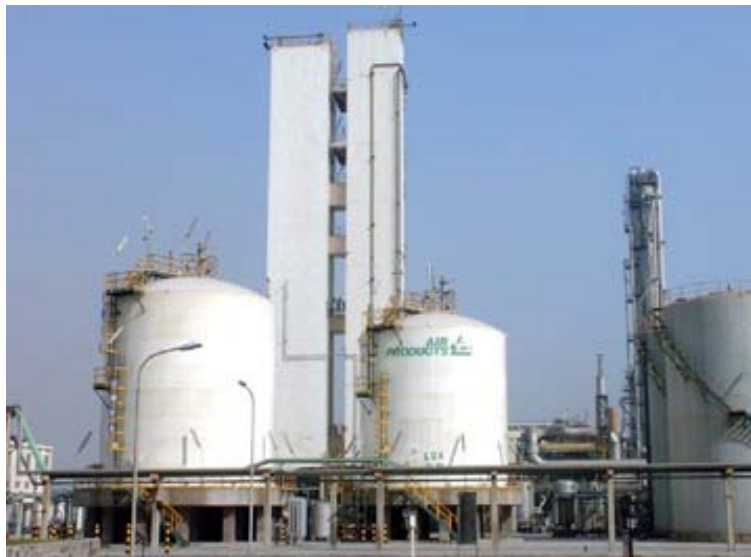
Figure 2 Cryogenic air separation plant with heat exchanger and distillation column towers (source Air Products)
