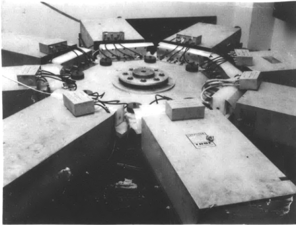
Photo 1 Capacitor bank and transmission line.
