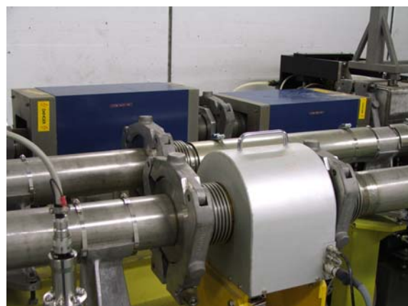
Fig. 10: A current transformer installed in the beam line
