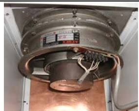
6.6 – Top side fan used to exhaust warm air from enclosure.
