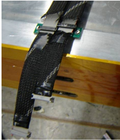
Figure 17: RPC 'cable stop'. Cable stops are installed close to the front-end cards on all cables going to the LV1 trigger boxes, to reinforce the RPC grounding scheme and improve immunity against noise.
