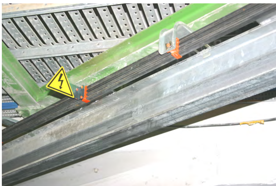
Figure 4.6: The FABA100 power rail mounted in the LHC tunnel, alongside the monorail
