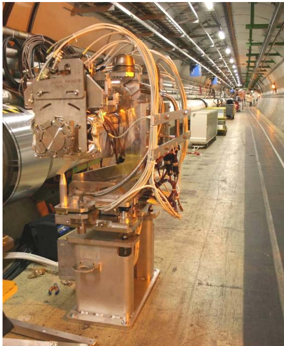
Figure 6: Photograph of an installed ring collimator on its quick plug-in support in IR8 of the LHC.
