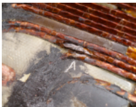
Fig. 10 Short circuit on the inside of the inner layer. The scratched arrow points to the spot between turn 3 and 4 on the connection side.
