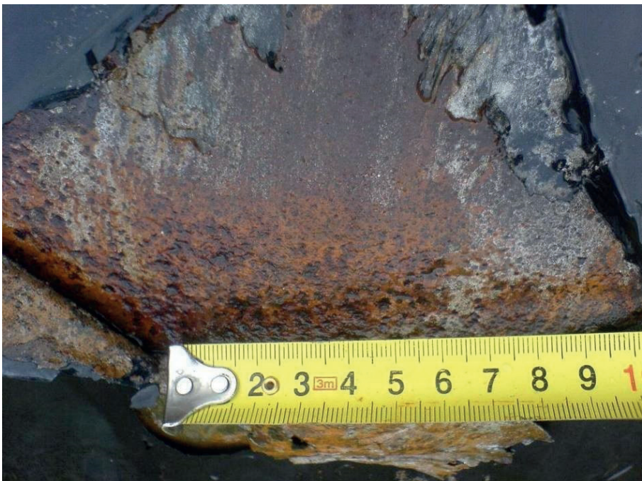
Fig. 5. Pitting corrosion of the metal of the gas pipeline
