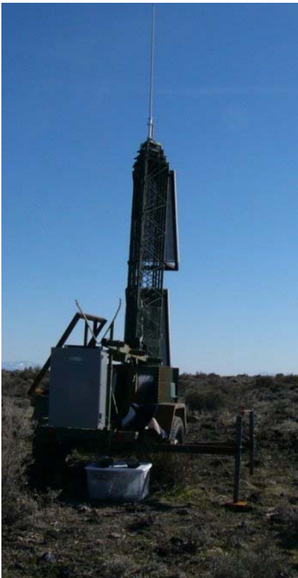
Figure 4. The communication tower. This is the tower setting temporarily. We will construct communication towers fixed ground. These are 15m heights and have the lift of directional antennas. Communication towers will set 5 places and they will be able to communicate each other.
