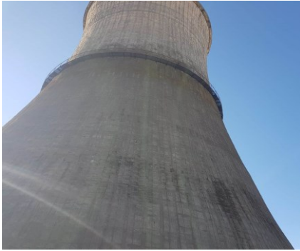
Fig. 3. Cooling tower body.
