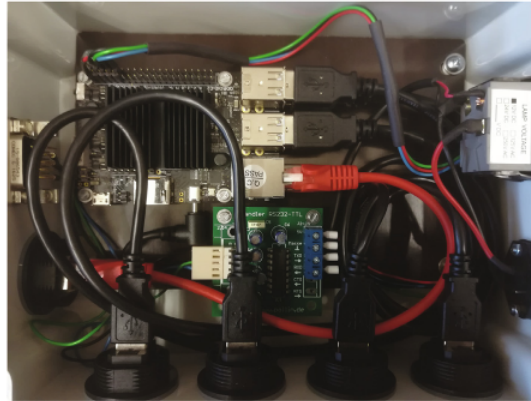
Fig. 13. The USB and Ethernet cables connected to the couplers.
