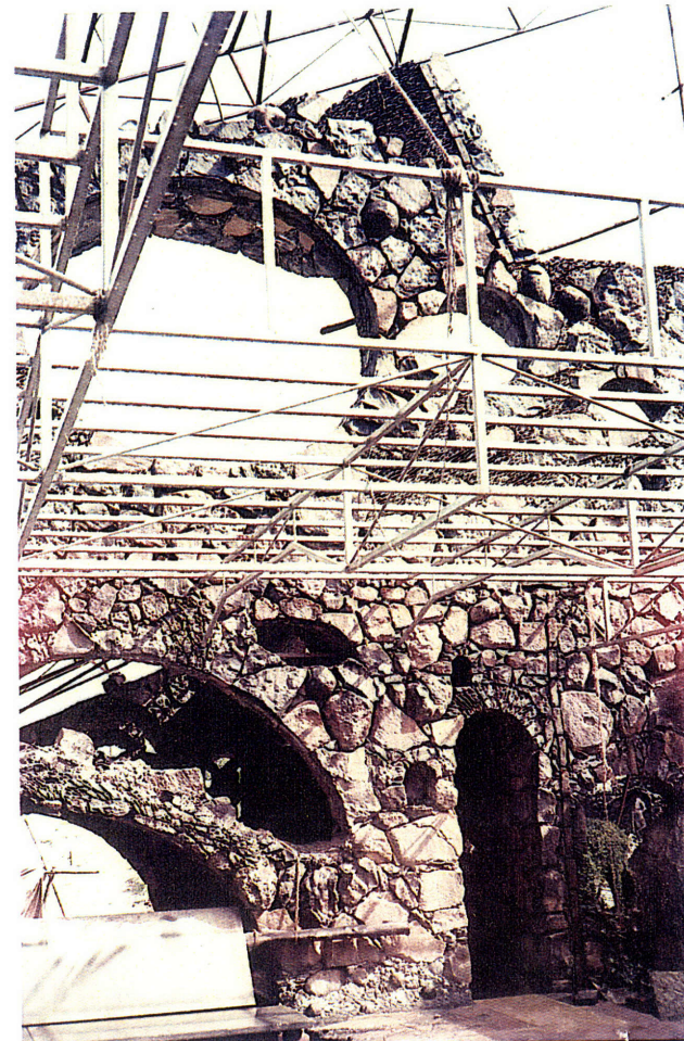
Left: Top, creepers dangle from the balcony platform and the walls, roofs are yet to be completed.
