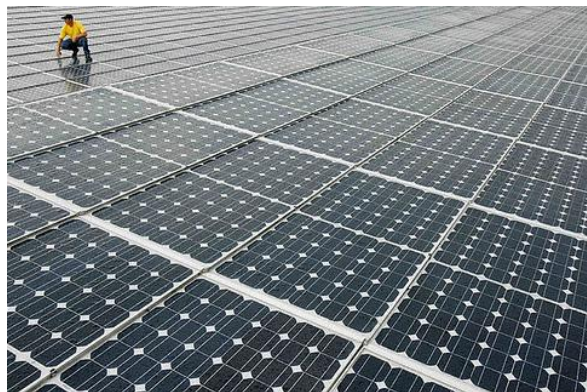
Figure 6: Large Photovoltaic Array
