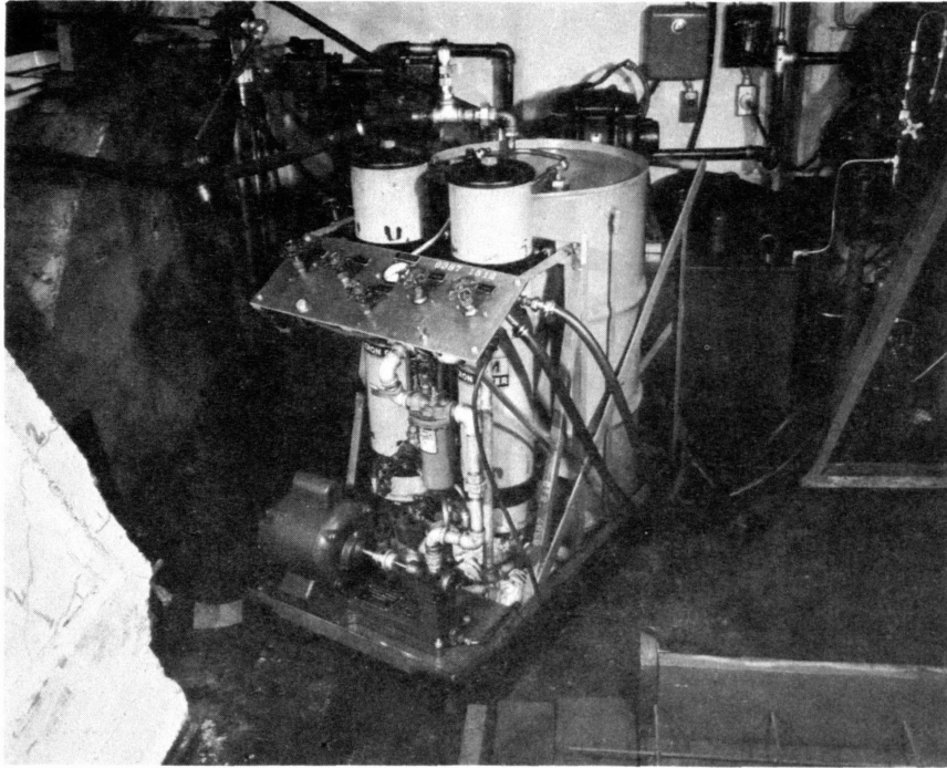
Figure 23 - General View of the Filter Unit
