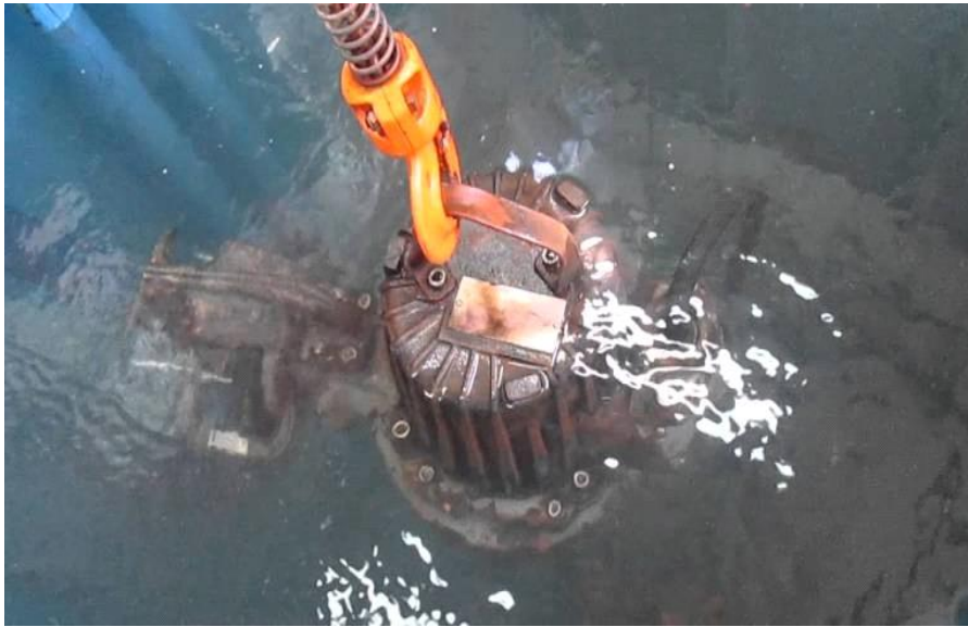
Fig. 3. Submerged wastewater pump
