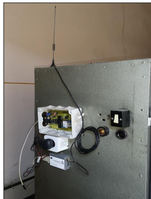
Fig. 7. Switch heating remote control device, mounted on a metal panel
